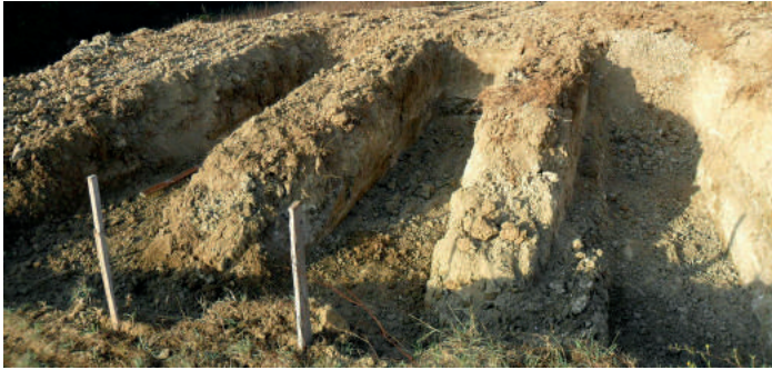
① EXCAVATION Dig a trench at least 900 mm wide at the base.
