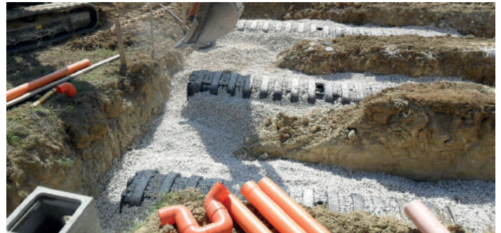
④ COVERING Connect feeing and ventilation pipes. Cover with at least 150-200 mm of gravel 20/40 mm.
