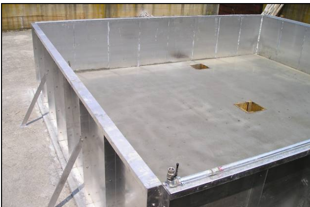
Fig. 3 Biofilter with metal walls
