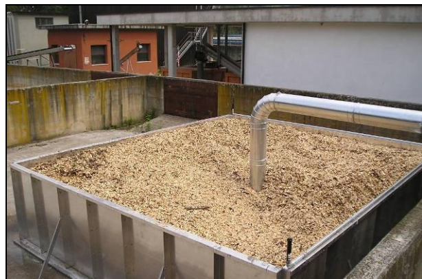
Fig. 4 Filter in use
