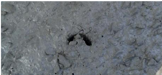
Figure 57 - the impression in the concrete indicates the right time to resume the casting
